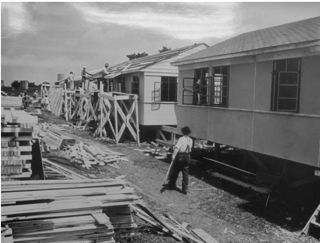
Image #19: TVA Outdoor Prefabrication Site (TVA Archive, National Archives Building, Atlanta, GA.)
