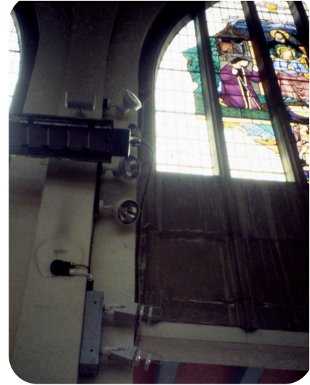
Bad installation of mechanical and electrical in a Victorian church
